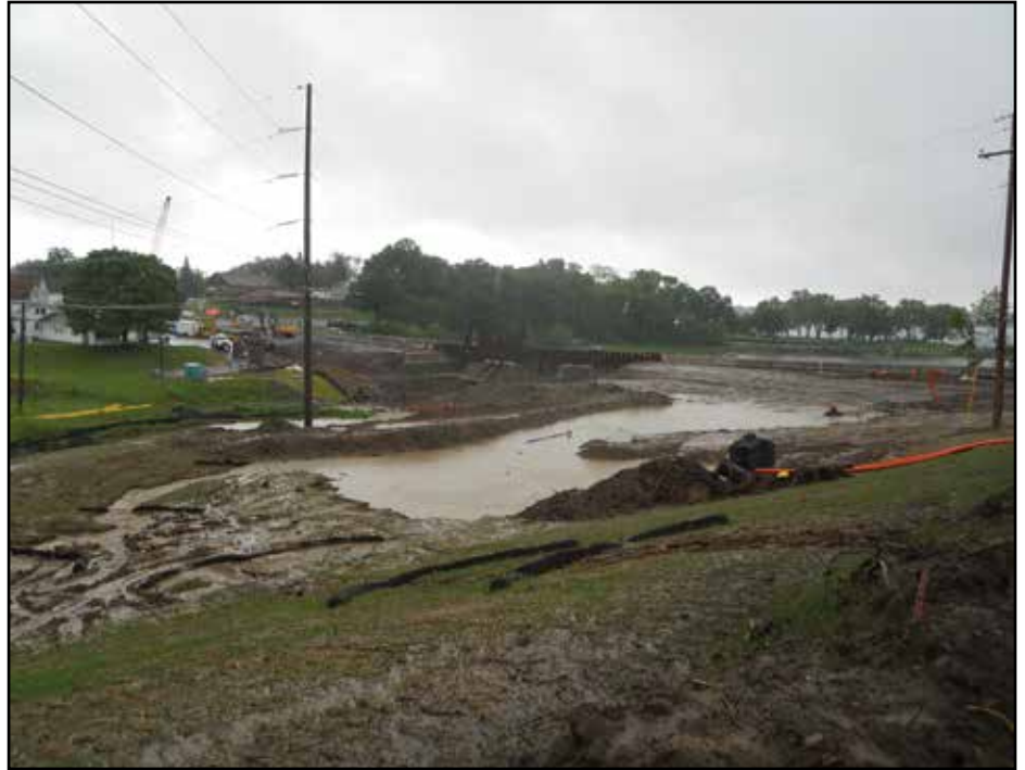
Conducting site inspections during and after rain events are useful in determining where attention needs to be focused and SWPPP modifications needed.
